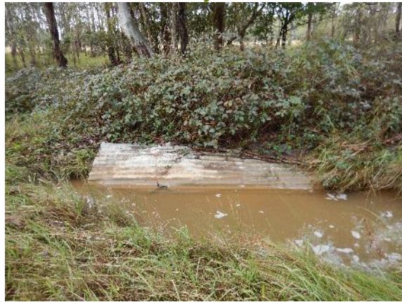
Plate 4: Debris washed into area after recent heavy rains
